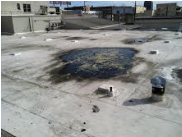
This conventional roof provides no human health or environmental benefits, while it creates a heat island and an ugly view for adjacent building dwellers.
