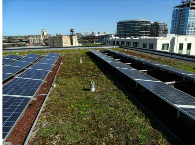
The Ramona Apartments' roof elegantly and efficiently combines solar panels and an ecoroof creating an attractive view, energy savings, habitat, and cooler, cleaner air quality.
