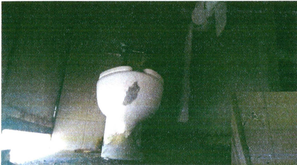
Pier Park toilet, women's side. Note rust on wall.
