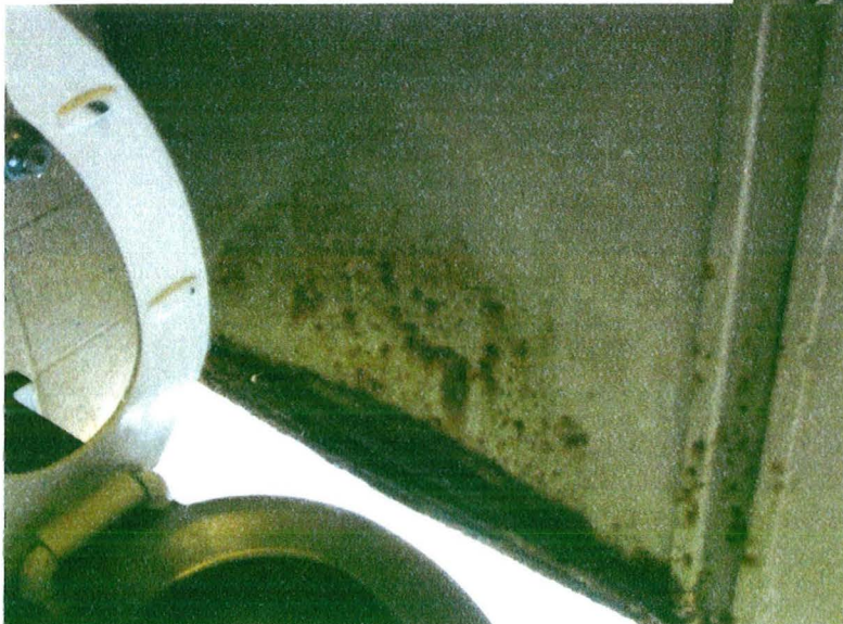
Pier Park toilet, men's side. That is rust growing up the side of the "tin palace."
