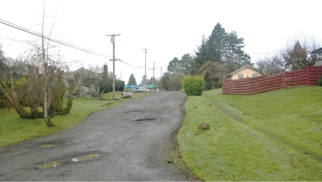
SW Carson Street, east of SW Terwilliger. A severely under-improved and narrow roadway.
