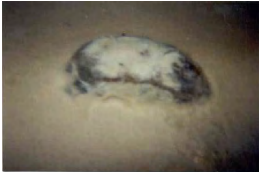
Deceased rat on layers of sediment in a covered reservoir. Common entry points for rodents, cats, and birds in covered reservoirs are hatch or access openings, vent pipes, structural cracks, and overflow pipes. (Ref. 58)
