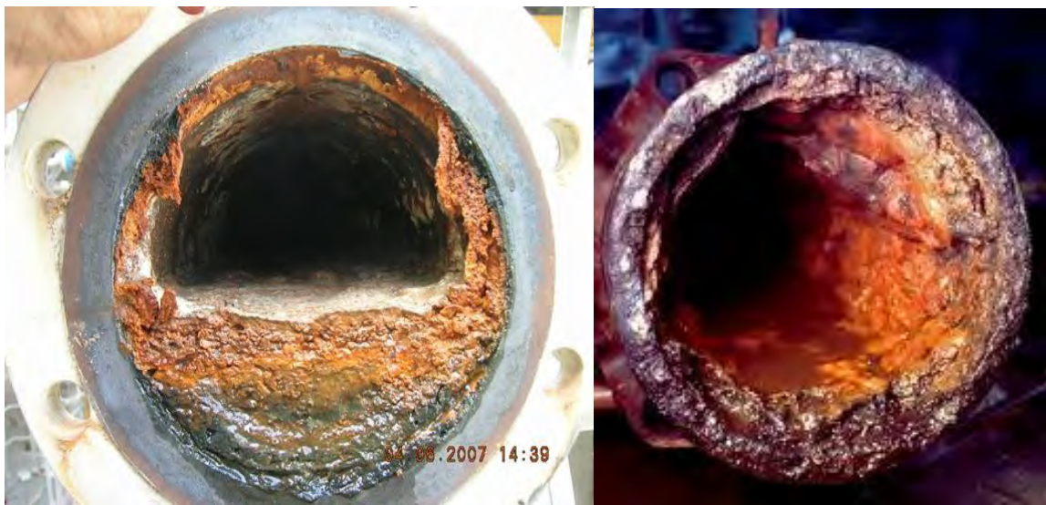
Example of water pipeline biofilm & sediment accumulation from years of Portland Water Bureau deferred maintenance and system neglect as source of alleged contamination resulting in “boil-water” notice on May 23, 2014
