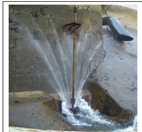
Figure 39. Third outlet pipe in Reservoir 1 next to the gatehouse on the north side.
