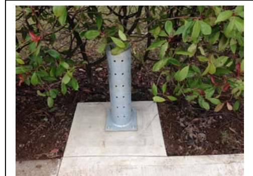
Figure 24. Example of air vent pipe.
