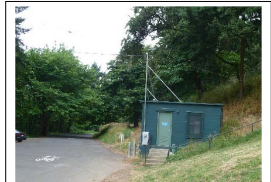
Figure 11. Electrical conduits in Work Areas 3 and 4 will connect to existing electrical system in the 44-inch meter house.
