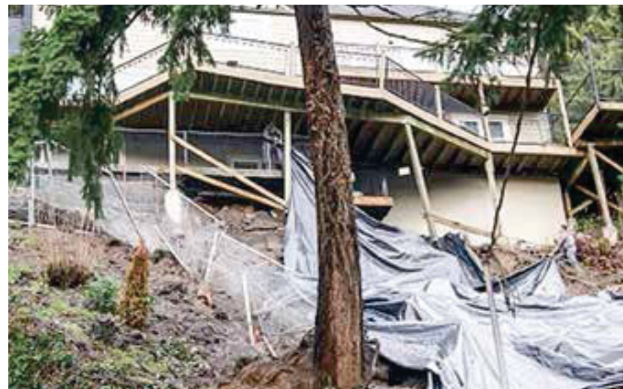
Landslides in Portland are a particular problem for roads and houses in the West Hills
