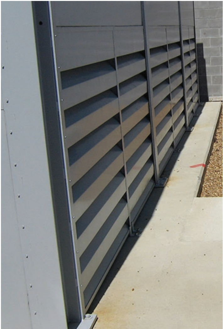
Acoustic Louvers at Cooling Towers
