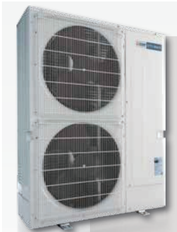
Split System Heat Pump - East Building
