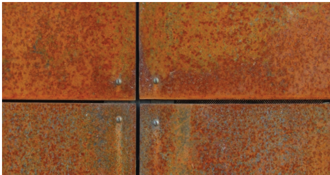
Weathering Steel Plate Fire place
