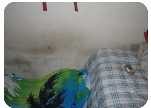
Keeping furniture and other belongings at least three inches away from walls will help prevent mold like this from growing.
