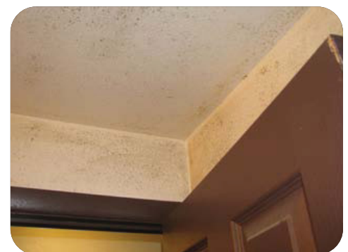
Mold consultants can contain and treat this spreading mold problem.
