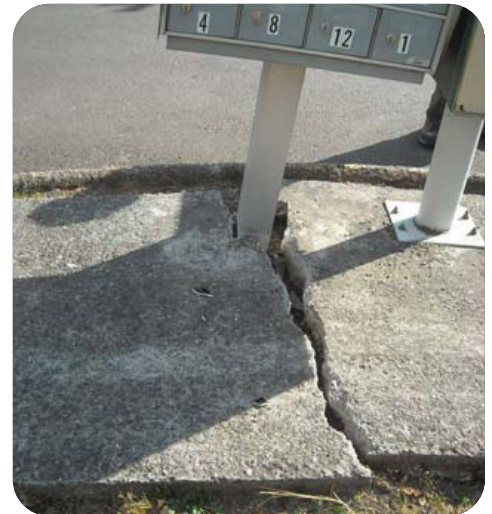
Cracks in sidewalks present trip hazards and project the wrong image.
