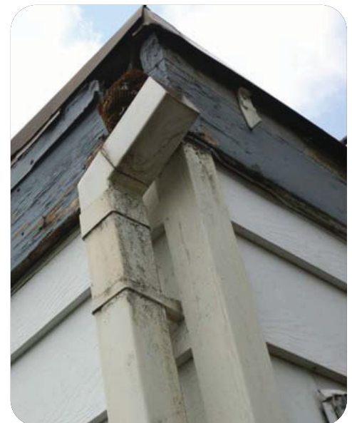
This roof has no gutter, so the downspout is clearly not serving its purpose.
