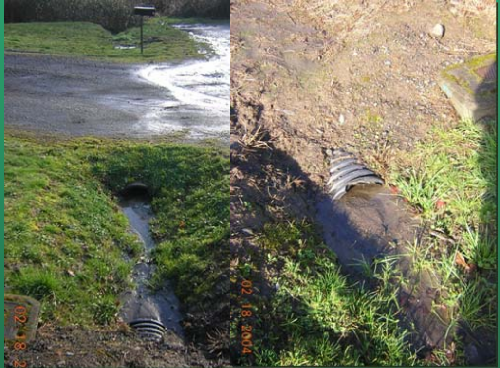
Drainage ditches clogged by eroded sediment
