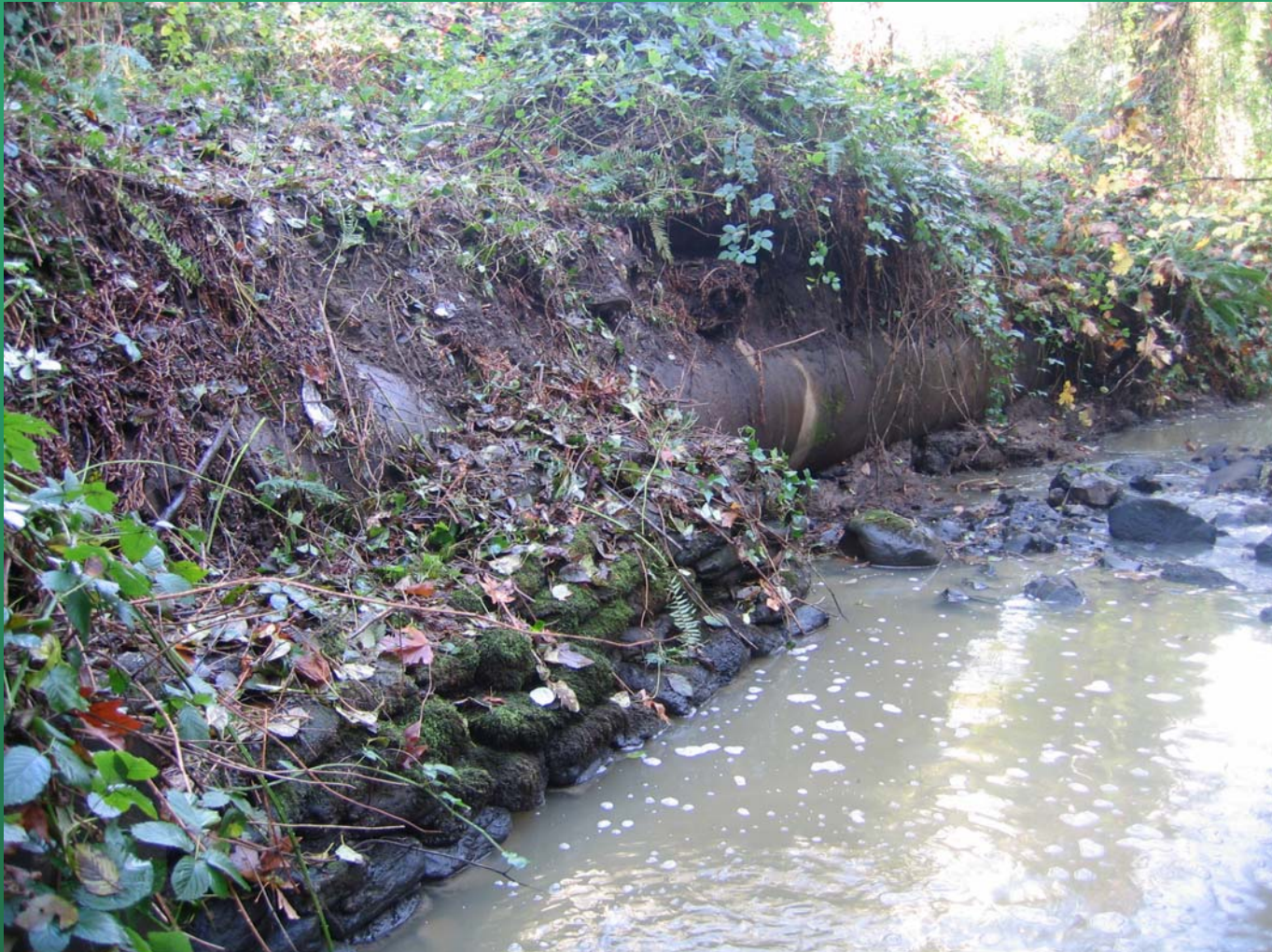
Burlingame line paralleling Stephens Creek, exposed by stream erosion
