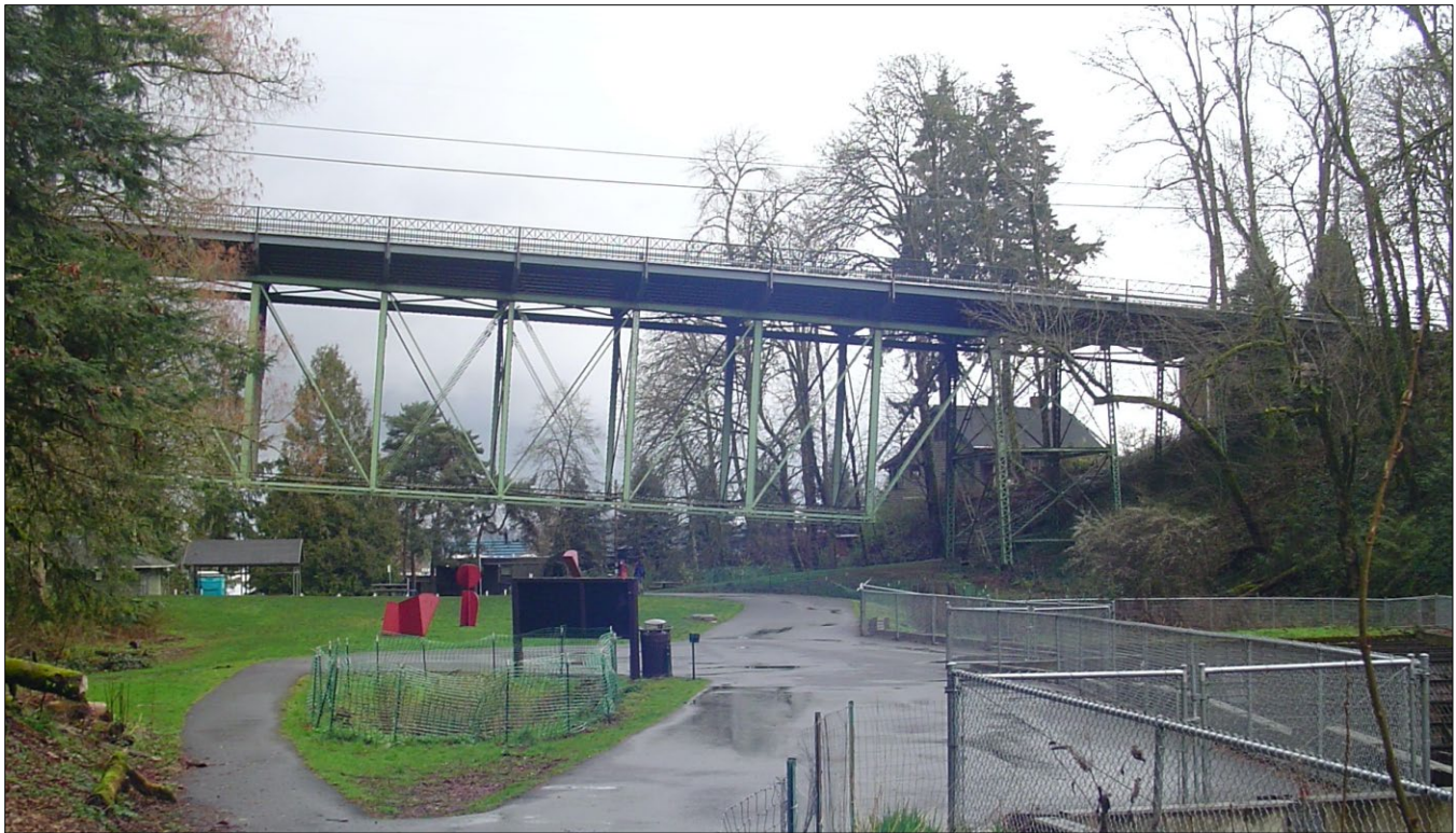
Photograph 1 of 12: OR_MultnomahCounty_BalchGulchBridge_0001 Eastern portion of the Balch Gulch Bridge including 160' deck truss, looking north from Lower Macleay Trail.
