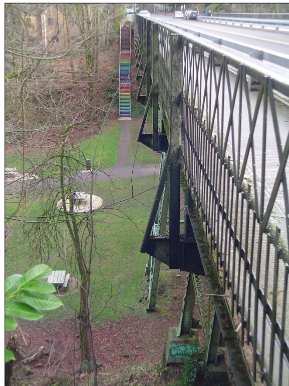
Photograph 2 of 12: OR_MultnomahCounty_BalchGulchBridge_0002 North side of the Balch Gulch Bridge, looking east from the northwest corner of the bridge. The staircase, which was initially constructed in 1950, is a separate structure.
