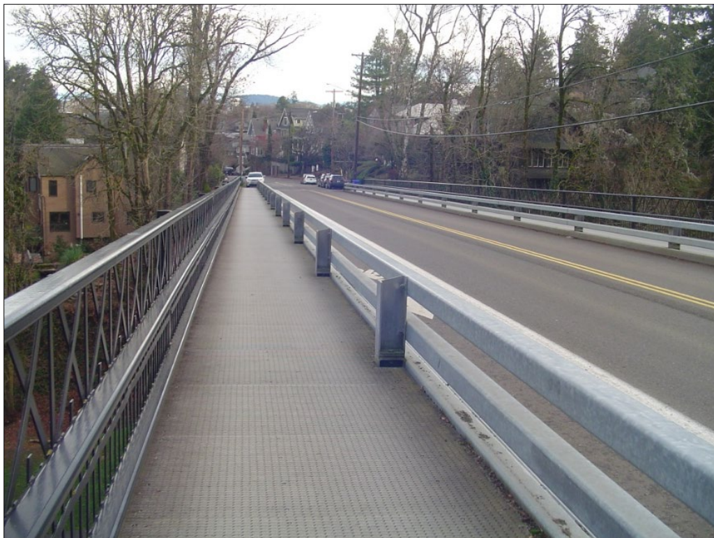
Photograph 4 of 12: OR_MultnomahCounty_BalchGulchBridge_0004 Balch Gulch Bridge deck, including reconstructed railing and replacement corrugated metal panel walkway, looking east from the northwest corner of bridge.
