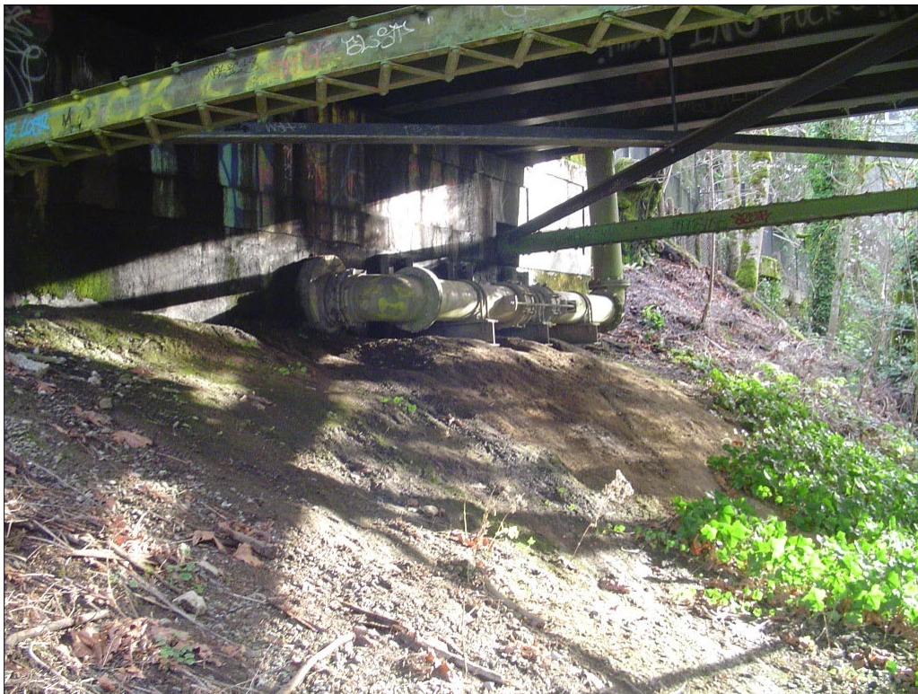
Photograph 12 of 12: OR_MultnomahCounty_BalchGulchBridge_0012 Underside of east concrete abutment footing, showing water main pipe, looking southeast.
