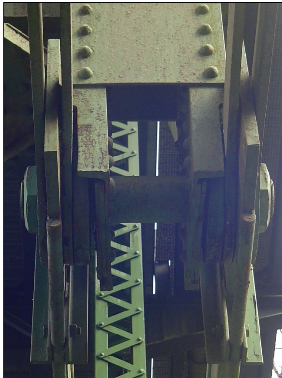
Photograph 10 of 12: OR_MultnomahCounty_BalchGulchBridge_0010 Detail of pin connection on southwest corner of 160' deck truss, looking upward/east.
