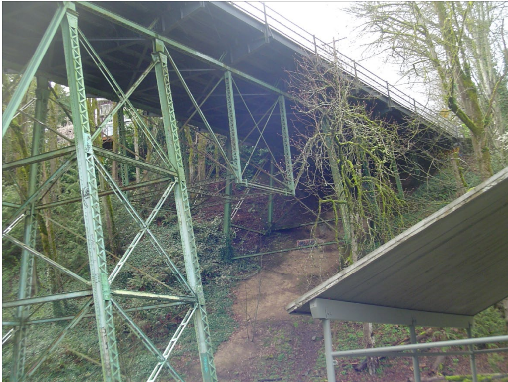
Photograph 7 of 12: OR_MultnomahCounty_BalchGulchBridge_0007 Detail view of 60' deck truss at the western side of the Balch Gulch Bridge, looking southwest.
