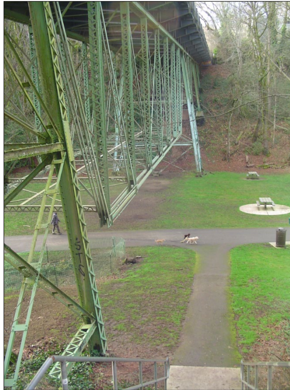
Photograph 5 of 12: OR_MultnomahCounty_BalchGulchBridge_0005 Balch Gulch Bridge trusses, looking west from the staircase in the hillside at the northeast corner of the bridge.
