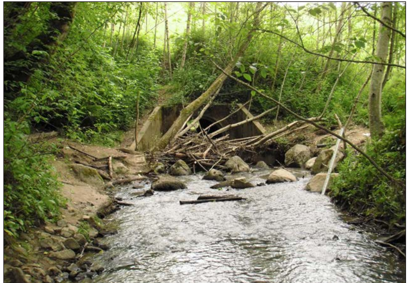
The Cedar Mill Creek site shows wood and boulders piling up at a culvert. Culverts often limit the passage of large wood and fish and wildlife and degrade stream flow and water quality, which adversely affects stream health.
