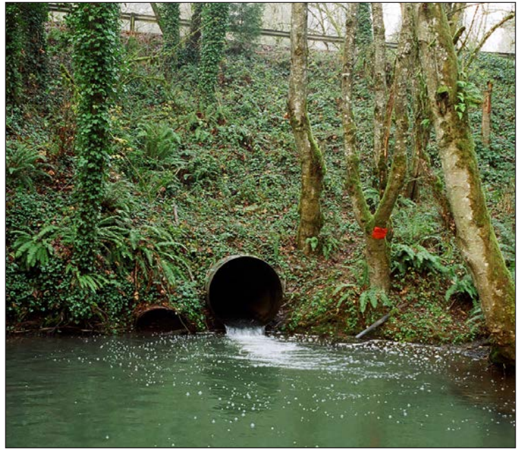
Culverts, like this one on Tryon Creek at SW Boones Ferry Road near SW Arnold Street, impair fish by blocking passage to some of Portland's highest quality fish habitats.
