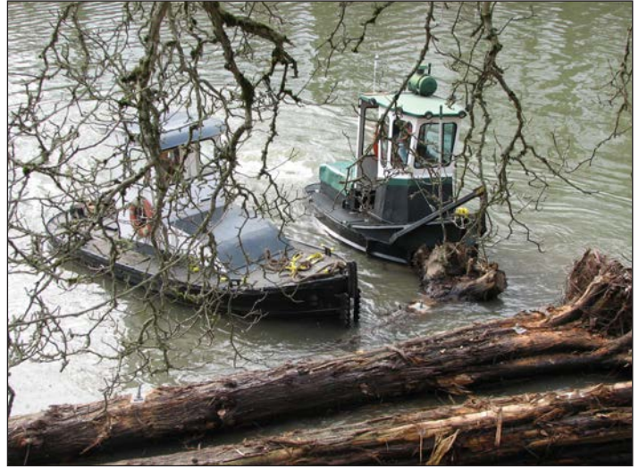
Restoration projects like the Lower Columbia Slough Refugia Project add in-stream wood using boats, cranes and barges. The logs improve habitat without impacting existing natural resources or the slough levee.
