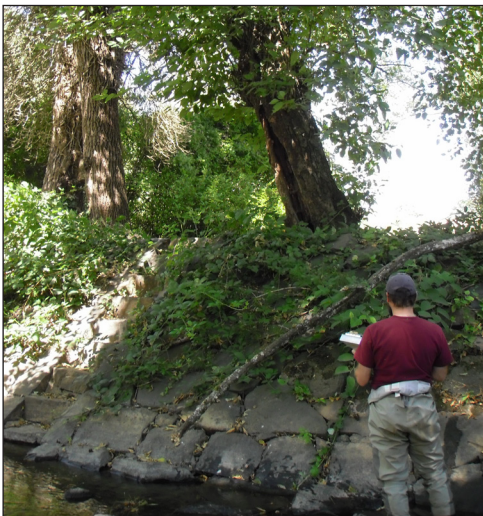
In the 1930s, the Work Progress Administration (WPA), deepened, straightened, and armored the creek by installing large basalt rock lining along its banks and streambed. The WPA work eliminated aquatic habitat such as riffles, pools, and large wood and impaired the stream's ability to migrate and recruit gravels and large wood. It also disconnected the stream from its floodplain which previously absorbed, stored, and conveyed floodwater.
