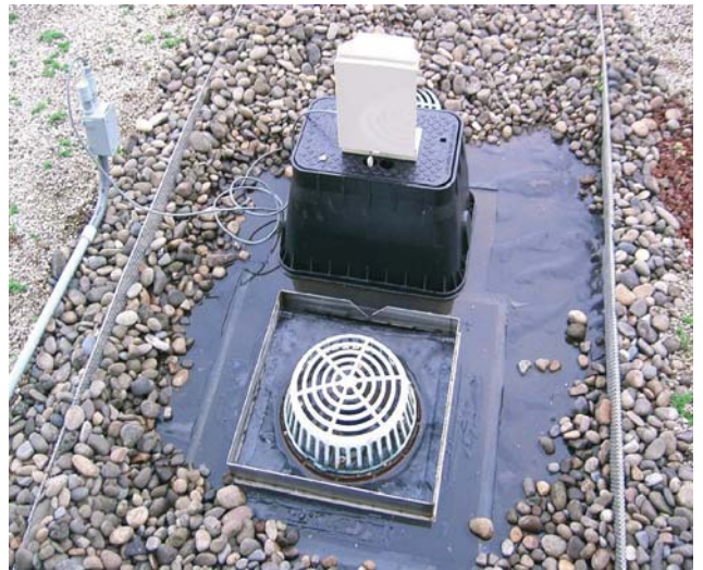
Metro Ecoroof Monitoring Equipment at the Roof Drain
