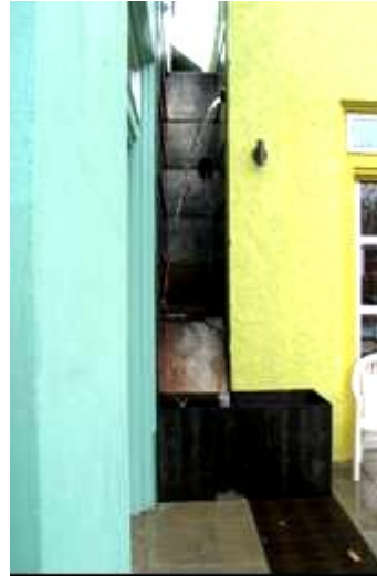
Downspouts disconnected to collection basin and conveyed along a trench to the planter
