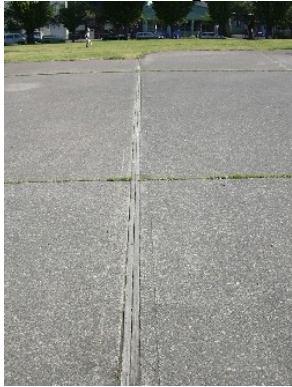
Figure 5: Wooden expansion joints
