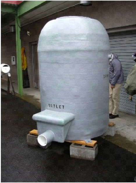
Manhole for accessing monitoring equipment
