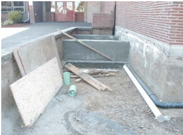
Figure 3: Monitoring, flow-through, and infiltration cells of stormwater planter retrofit (from back to front of photo)
