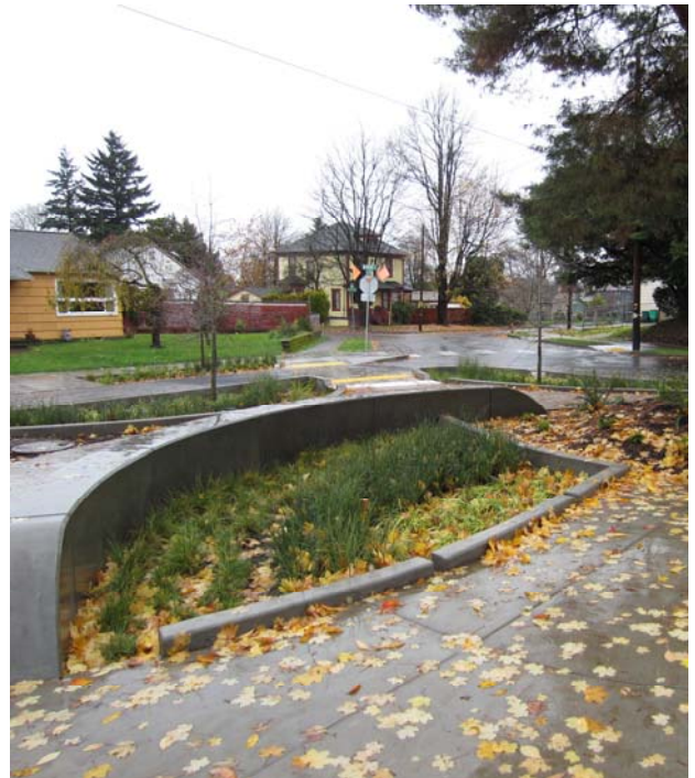
The infiltration planter also accepts runoff from the plaza inside Holman Park. It has a flat bottom and a ponding depth of 6". The site has extremely high infiltration rates. An emergency overflow pipe was installed, but has been left capped.
