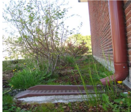
Figure 5: Disconnected downspouts in stormwater planter
