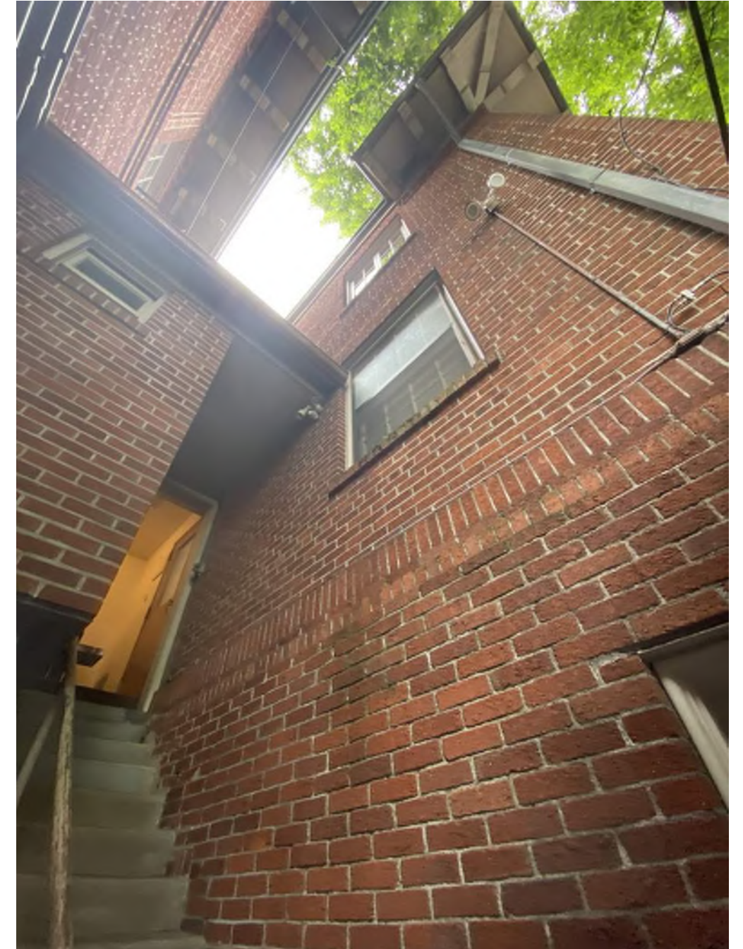
LOOKING UP AT ORIGINAL 'CLIPPED EAVES' OF THE NORTH BUILDING IN 'RAT'S ALLEY'
