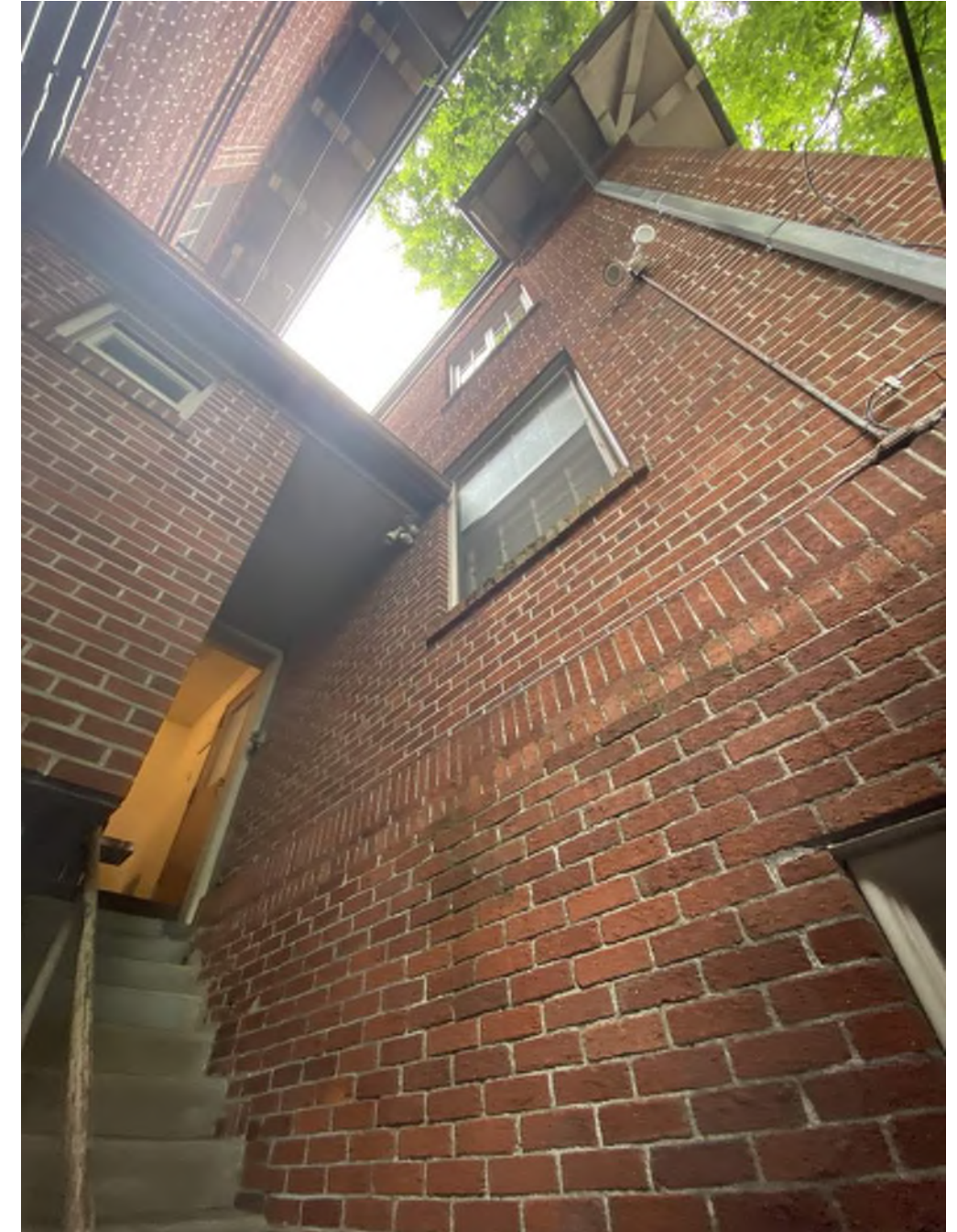
LOOKING UP AT ORIGINAL 'CLIPPED EAVES' OF THE NORTH BUILDING IN 'RAT'S ALLEY'
