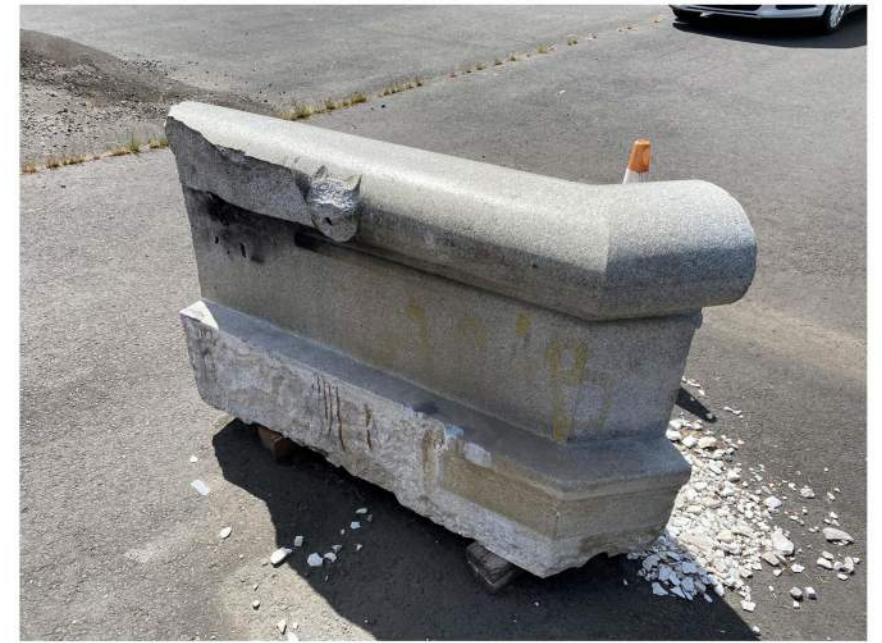
4 EXISTING BASIN WALL AT TROUGH SHOWN FOR REF OF MITERED DETAIL AT TROUGH
