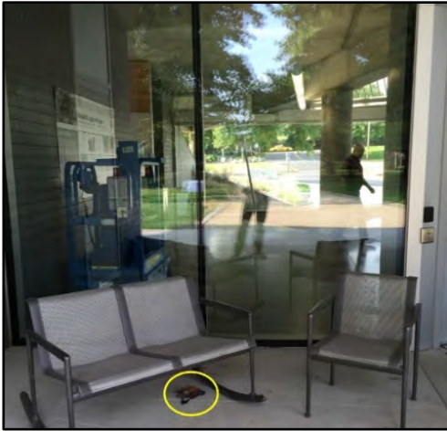
Photo 3: Example of the fly through hazard created by the lobby windows. A car is visible on Columbia Blvd on the other side of the building. A window collision robin carcass lies under the bench.
