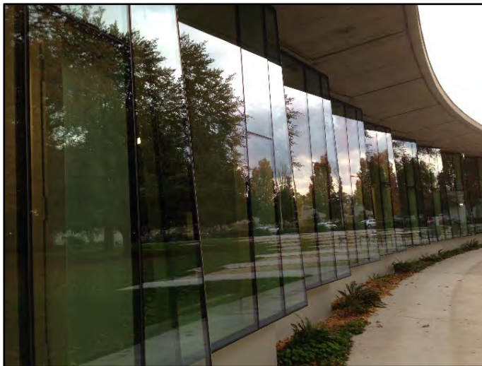
Photo 5: Another example of deceptive reflections creating a collision hazard on north-facing window banks.
