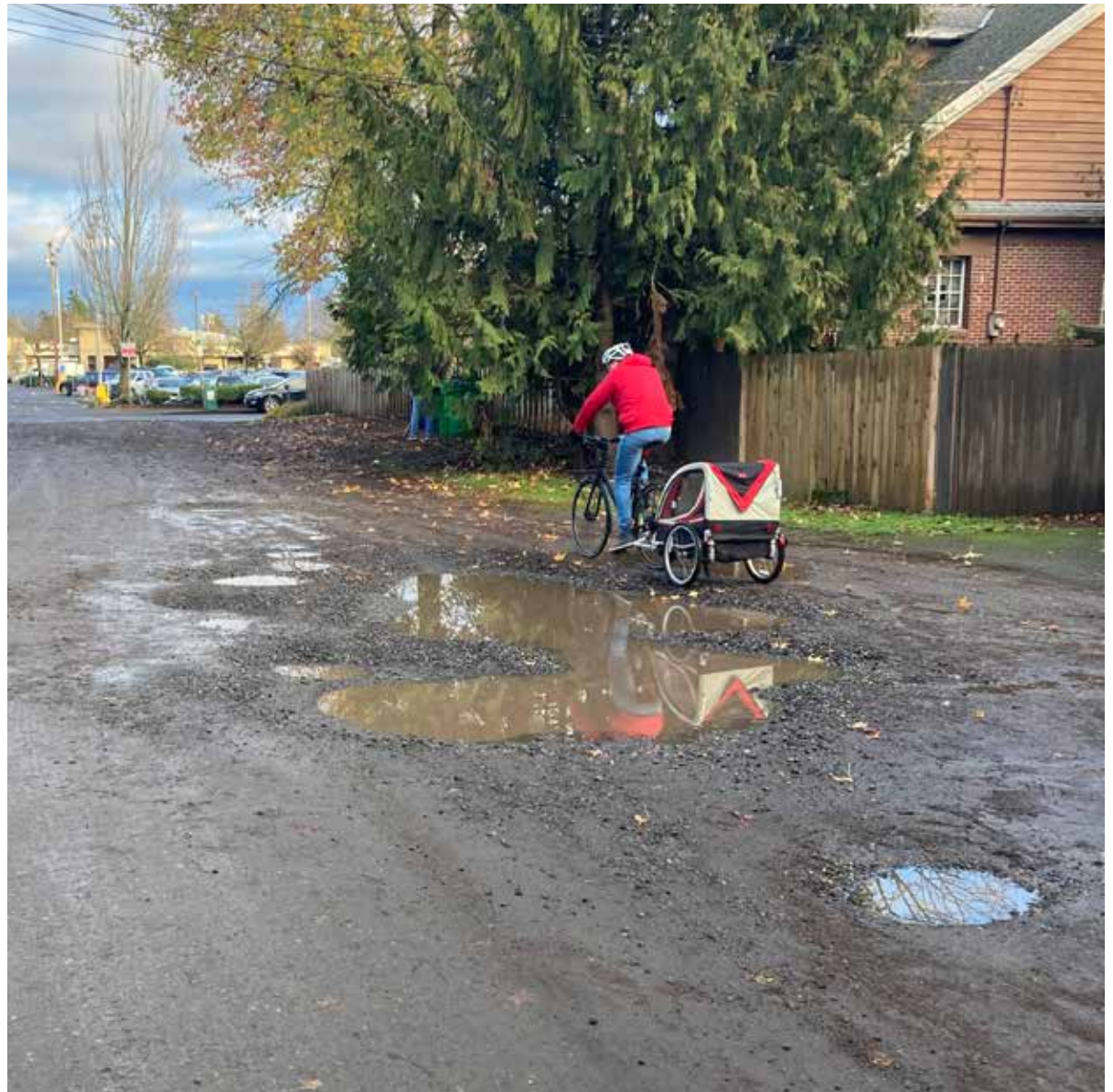
A cyclist navigates around water-filled potholes on an unpaved street in the Woodstock Neighborhood
