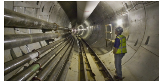
Inside the 14-foot diameter, 3.5 mile West Side Big Pipe, one of several City projects to control "combined sewer overflows" (CSOs).
