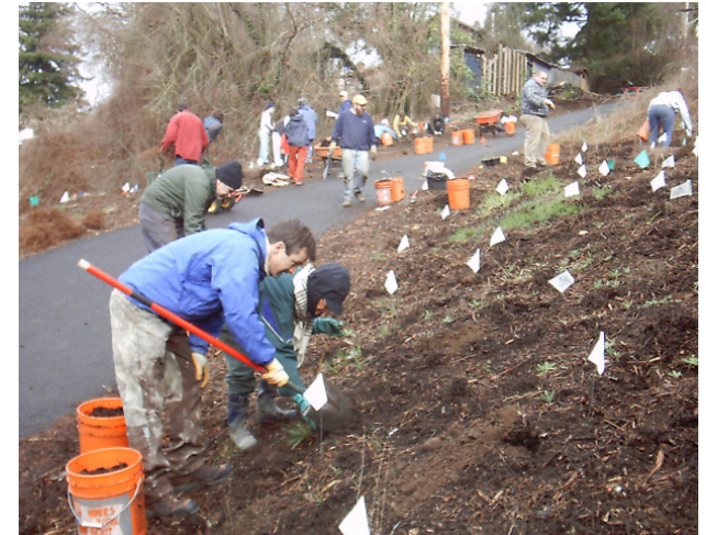
Community restoration work at Tideman Johnson Park during the Johnson Creek Watershed Council’s Annual Watershed-Wide Event. In 2008, about 400 volunteers participated in this event, planting over 6,000 plants. To date, BES has restored over 62 acres of Johnson Creek, its tributaries and its floodplain.
