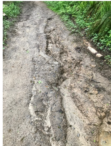
Erosion on Holman Lane
