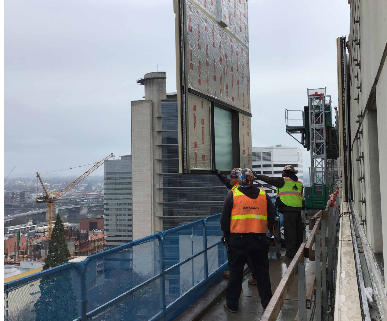
Unitized curtainwall panel being lifted into place over the original concrete building shell.
