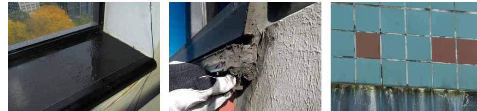
Photos documenting the building conditions prior to the reconstruction show evidence of the long-term water damage (bottom).
