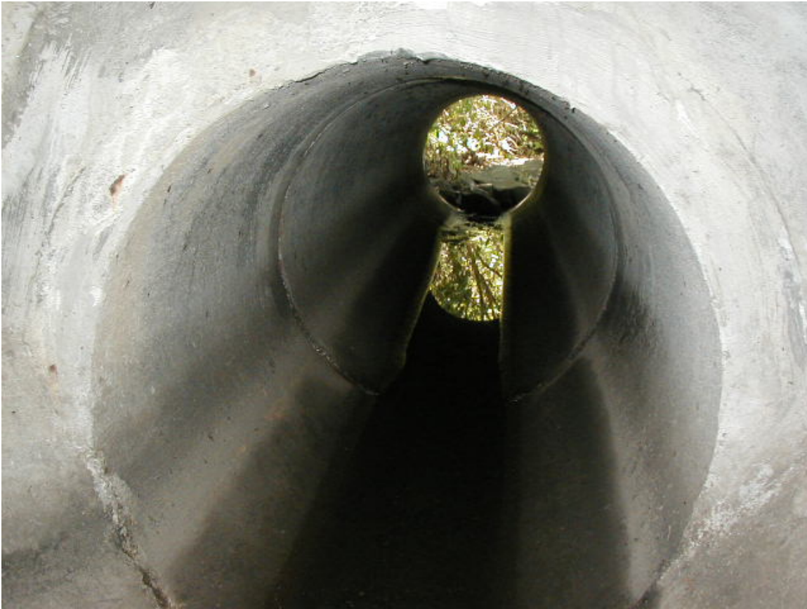
Photo 3 (July, 2005). Looking toward the drainage swale in Outfall Basin 49 from node AAG642. Solids were collected upstream from this location (see Photo 4).
