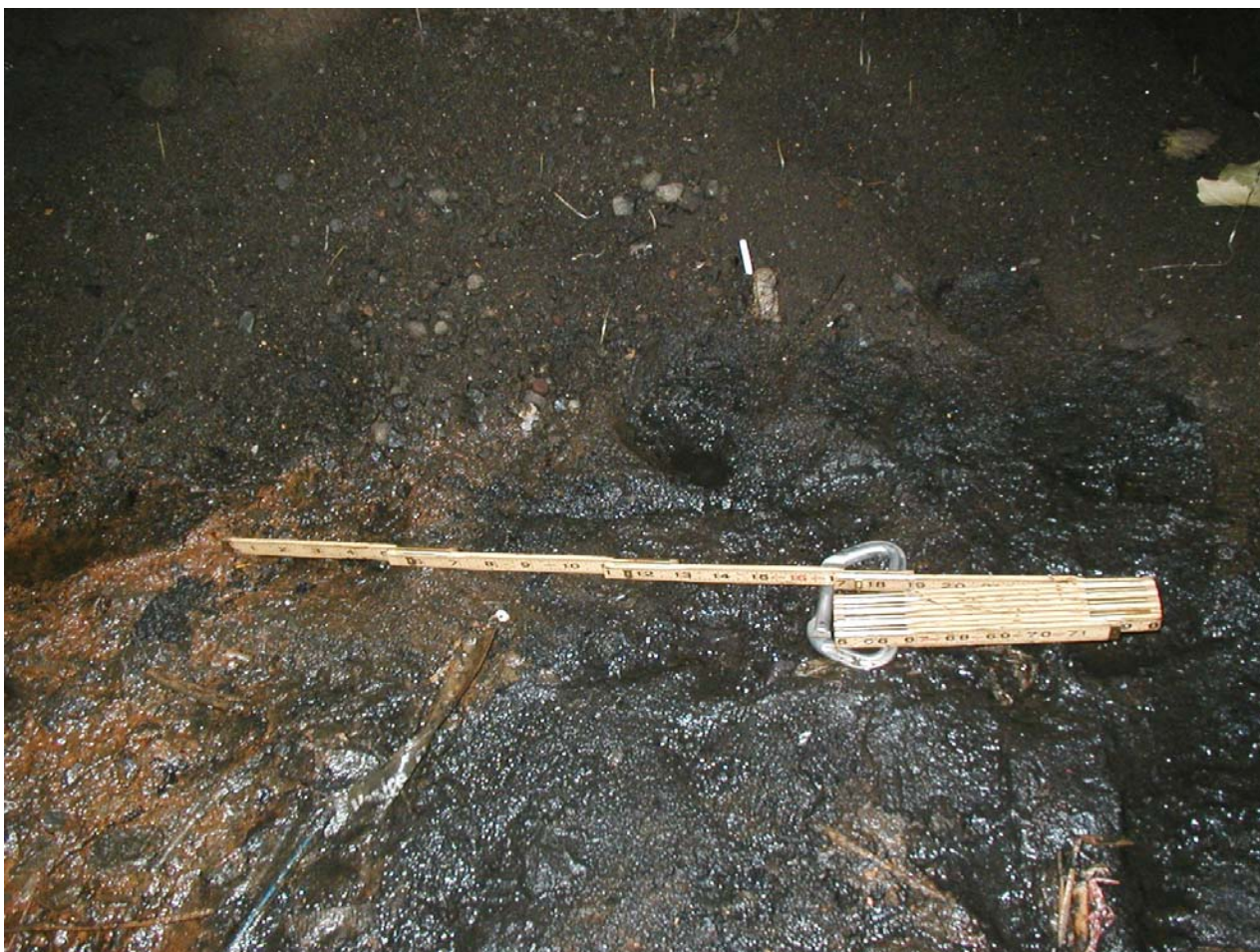
Photo 4 (June 2006). A solids sample was collected on this ledge, above the flooded floor of manhole AAQ090.
