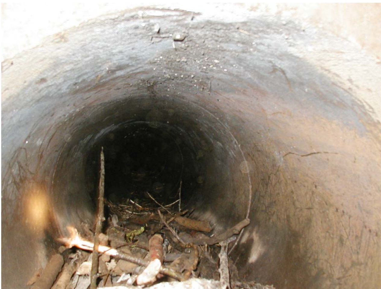
Photo 1 (June 2006). Looking downstream from manhole AAT623. Inline solids were collected at this location underneath the driftwood.
