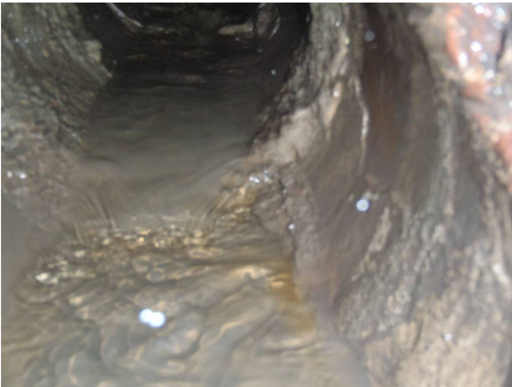
Photo 6 (March 15, 2012). Flow in 10-inch lateral entering Manhole ABC352 from the southeast.
