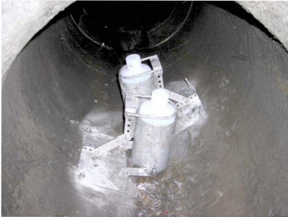
Photo 1. Inline sediment traps installed in lateral connection that discharges from the Calbag site to the City stormwater line in NW Kittridge Avenue. This photograph was taken during the installation of the Spring 2007 sediment traps. No photographs were taken during the installation of the Winter 2007/2008 sediment traps because of an equipment malfunction. Both sets of sediment traps were installed in the same exact location, shown in this photo.
