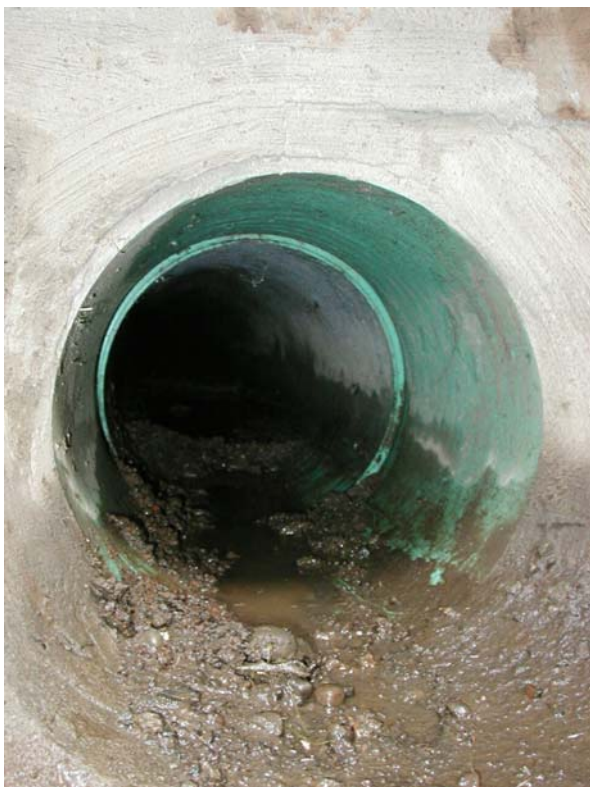
Photo 10 (August 2004): Inline solids from Wilhelm stormwater lateral ANB970, upstream of node ANB968.
