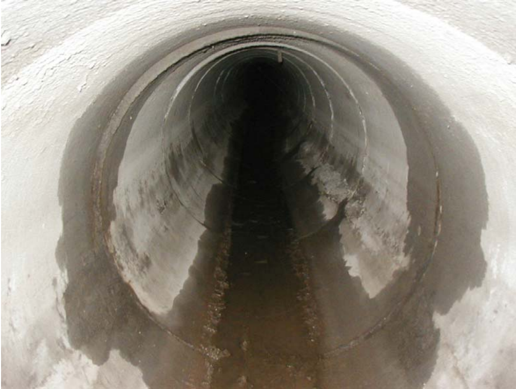
Photo 17 (August 2004): 42” stormwater line upstream of node AAX274.
