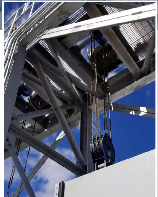
McMillen Jacobs designed the new hoist structure, which is over two bays, 21 feet tall, 50 feet long, and seven feet wide
