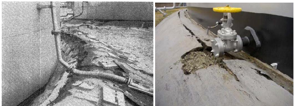
Figure 4: Liquefaction Induced Settlement following 1964 Niigata and 2011 Tohoku Earthquakes in Japan (Watanabe 1966, Zama et al 2012)
