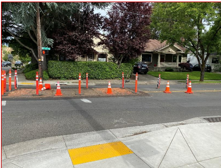
Photo 1: First sinkhole at NE 33 rd Ave & NE Knott (crosswalk on south side)
