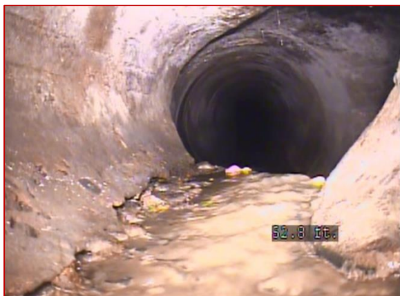
Photo 3: Deteriorated invert at 30"/60" junction, looking downstream 53 feet from AAY400
