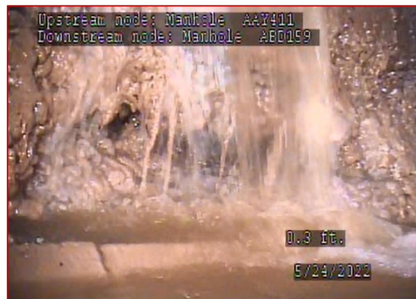
Photo 4: Scoured invert where 30" cascades to 66"
