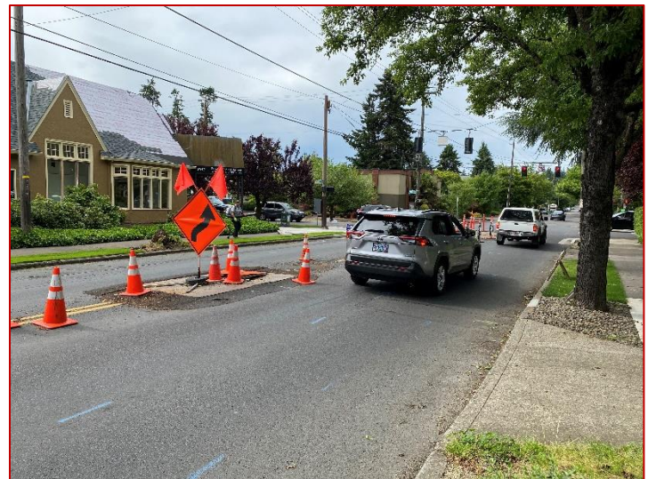
Photo 2: Second sinkhole on NE 33 rd Ave (approx. 60 feet south of first sinkhole)
