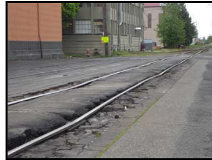
Poor pavement and rail conditions along N Bradford Street.
