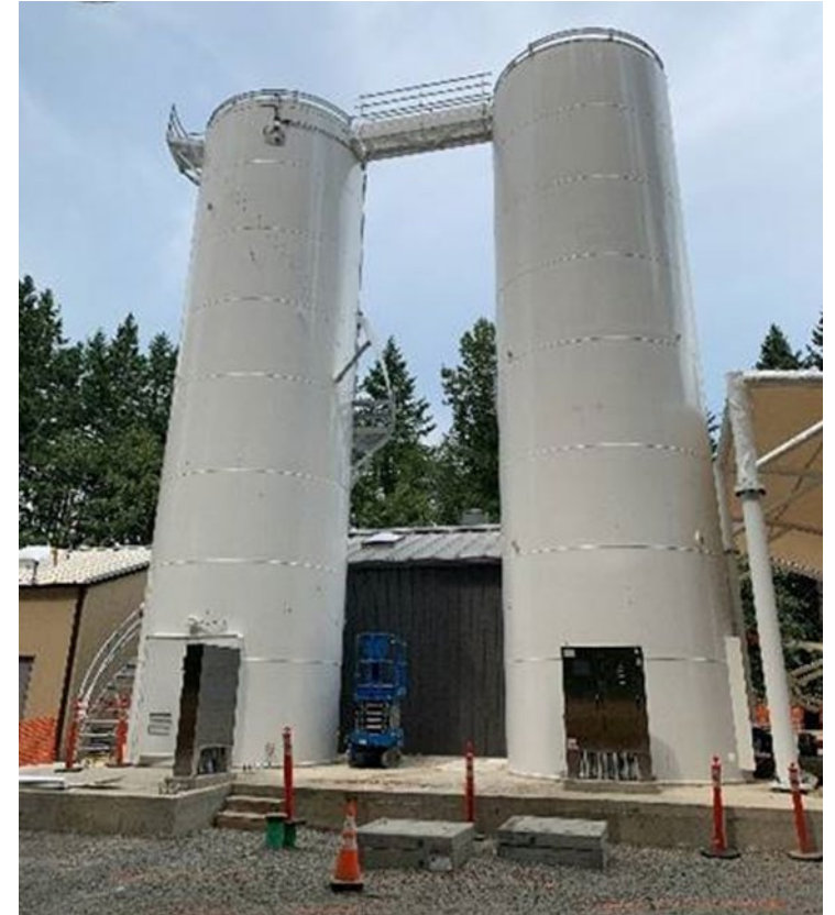
Soda ash silos recently installed at the Lusted Hill facility.
