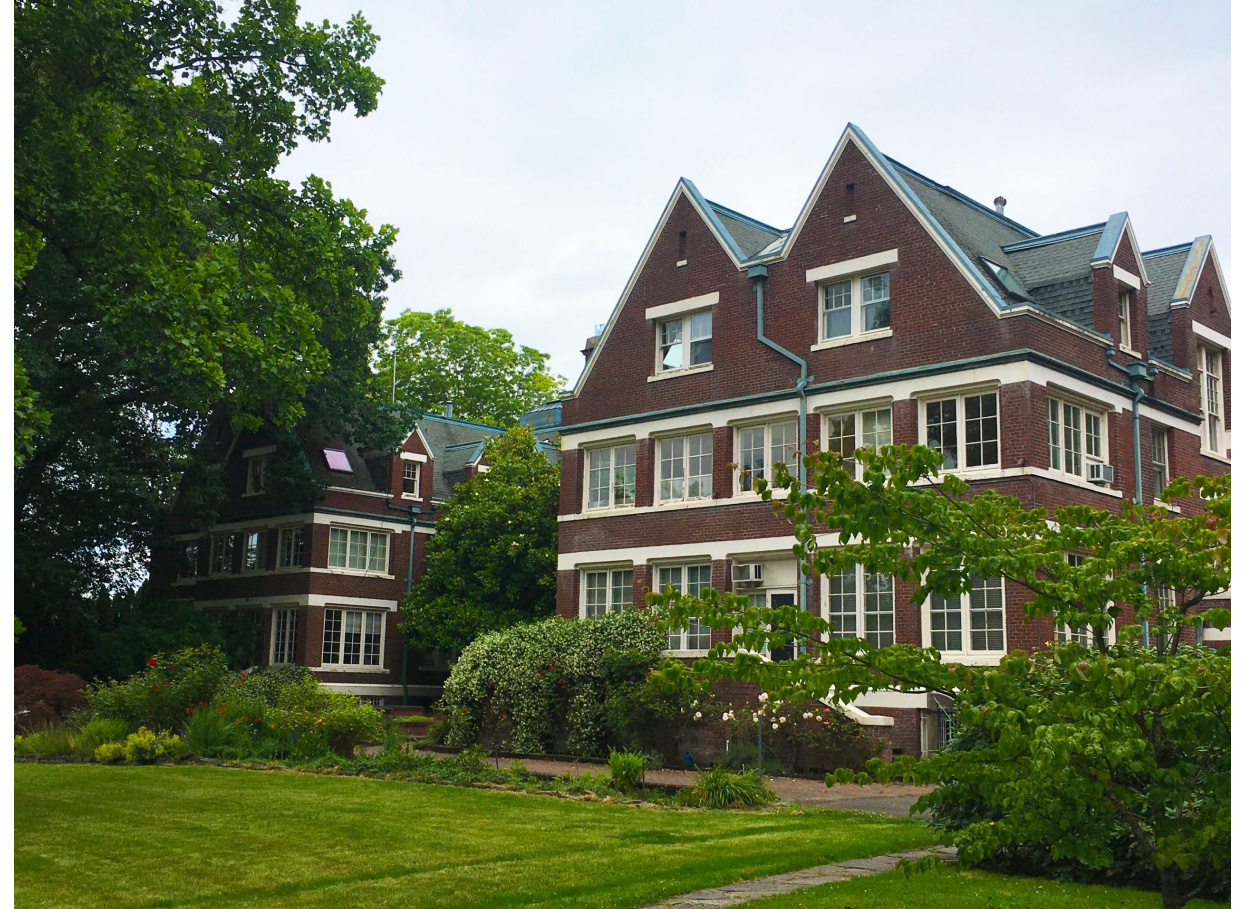
Anna Mann House, a Historic Landmark, currently undergoing rehabilitation for 129 family-oriented affordable housing units
