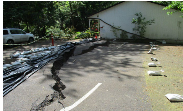
Example of an active deep landslide
