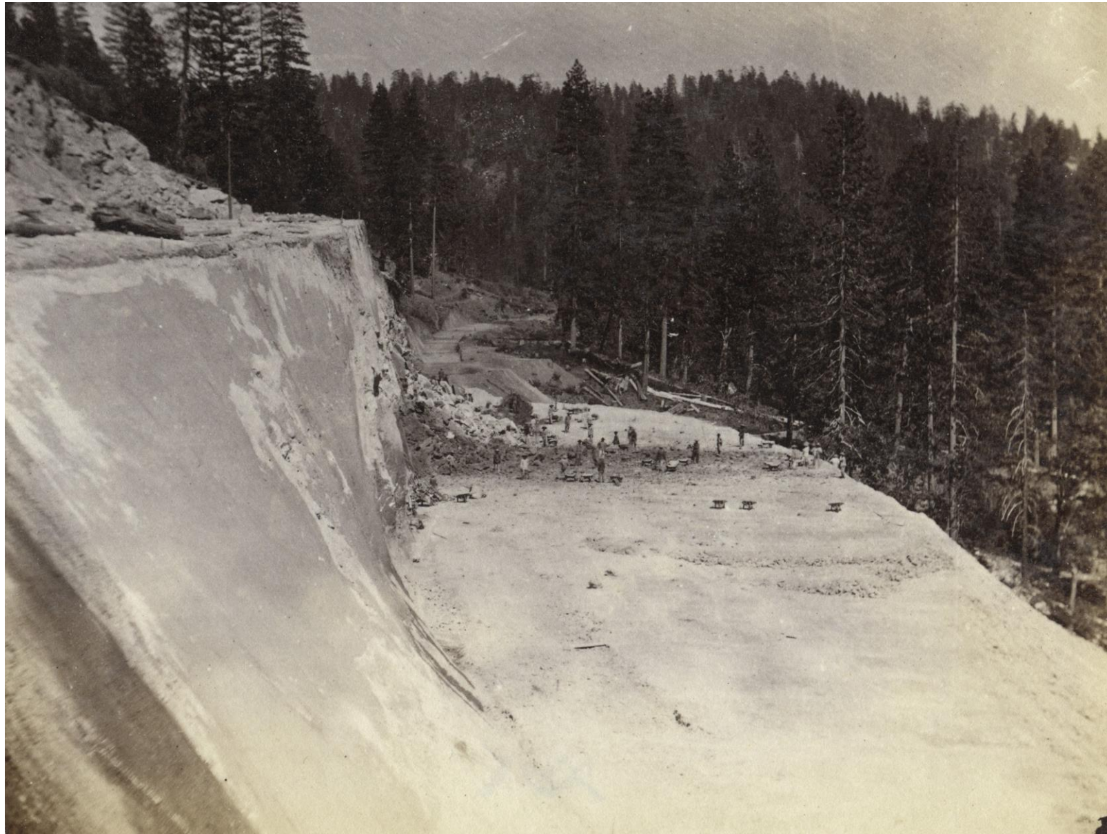
Workers blast a 60-foot-deep cut above Alta, California (1862-1869). Image credit: Hart, Stanford Univ.
