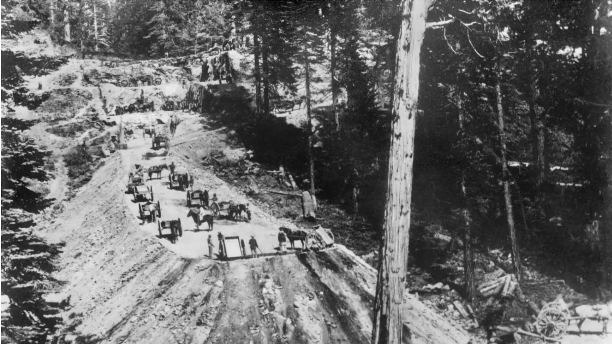
Chinese workers building a cut and a bank at Sailor's Spur in the Sierra foothills for the Central Pacific Railroad in California, 1866. Underwood Archives/Getty Images
