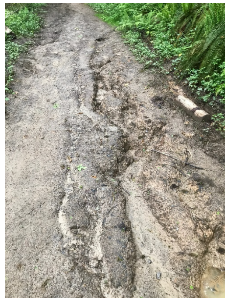
Erosion on Holman Lane
