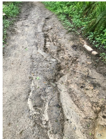
Erosion on Holman Lane
