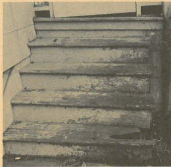
Steps leading to back entrance of house show need of rehabilitation.
