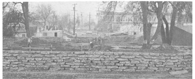
Woodlawn Park is beginning to take shape. An interesting pattern of rubble walls is being constructed using concrete from streets which formerly criss-crossed the park site. Upon completion of Phase I, the 8½-acre park will feature athletic fields, pedestrian walkways, small natural amphitheatre, picnic area, portable swimming pool, and play areas for tots and teenagers.
