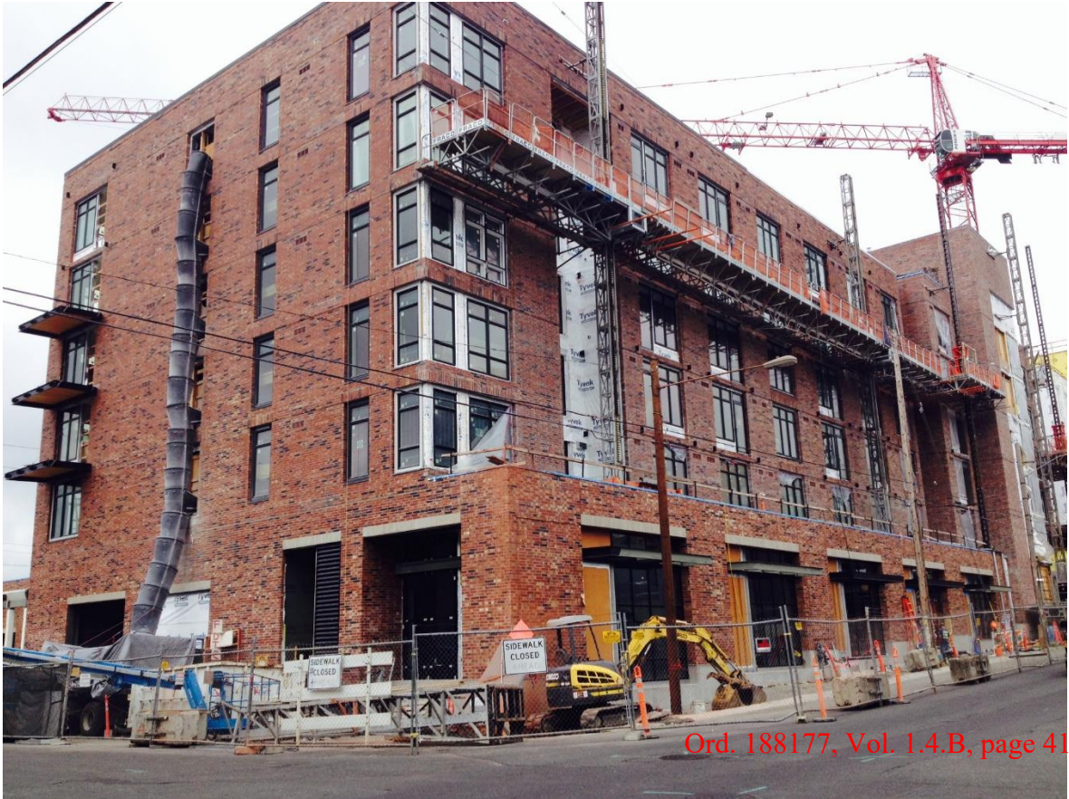
FIGURE 3 | STEPBACKS HELP COMPATIBILITY IN PORTLAND – Goat Blocks. Both images show better compatibility and density. Less box-like massing, stepbacks (in this case at the first floor instead of the third), varied window patterns, and brick in both Figure 2 & 3 creating better relationships to neighborhood patterns that keep the pedestrian scale and relationship to context while supporting more density above.
