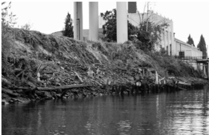
Figure 8: Abandoned pilings (Zone 3)
