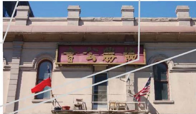
This Italianate building on NW 3rd Avenue retains its added upper-level awning, projecting sign, and fire escape. These alterations have acquired historic significance.
