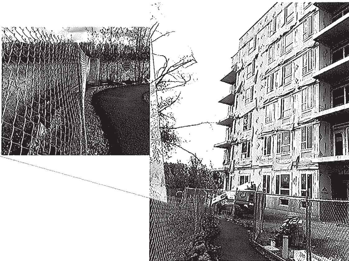
Current construction and greenway with 25' setback. Note how close trail is to building.
