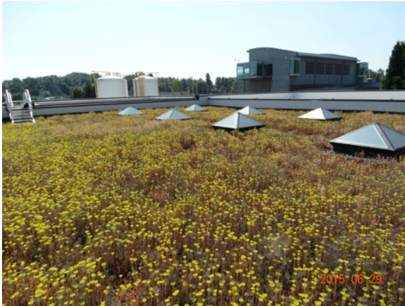
Figure 8 BES simple ecoroof at the Columbia Blvd. Wastewater Treatment Plant. It has no irrigation and the cost was $6 sf in 2011 when it was installed.
