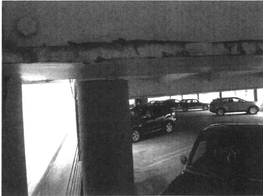
Figure 4, Evidence of rust in some steel sections
