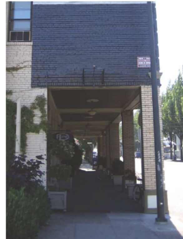
Burnside Arcade Condition
