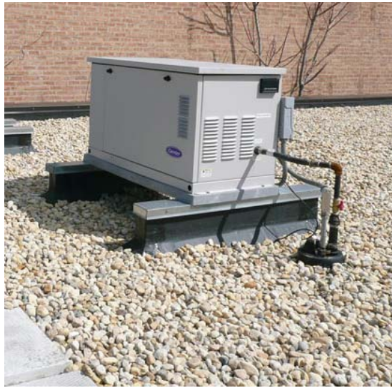
Example: Roof Mounted Generator
