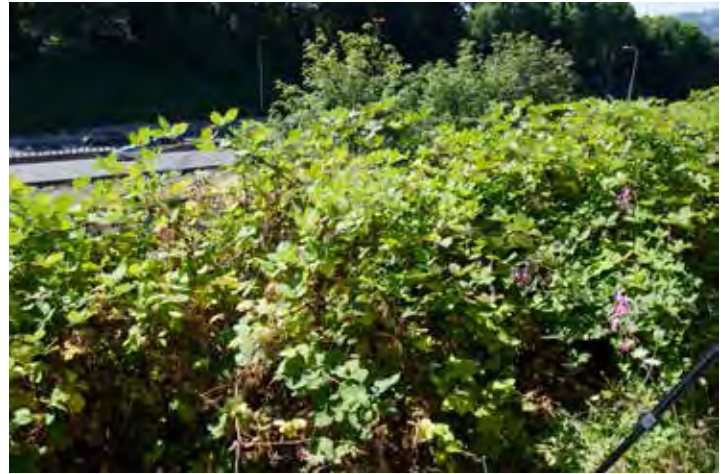
Overgrown vegetation at NE Lloyd Boulevard west of NE 9th Avenue
