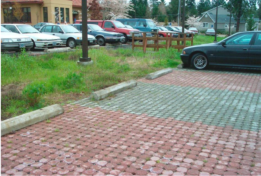
Exhibit 2-6: Multnomah Art Center Permeable Pavers. See Appendix G.1 , SW-110, for typical details.
