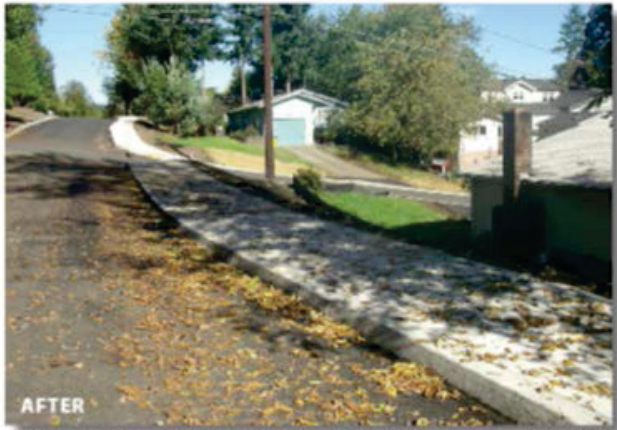
SW 28th Avenue South of Texas Street Looking North: After Substantial Completion of Construction
