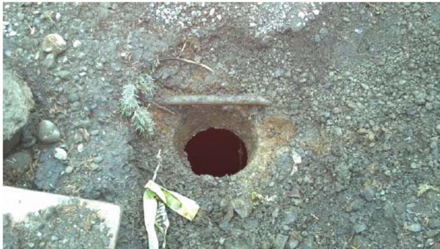
8 inch opening in concrete lid of buried UIC. The pipe visible in the picture is a natural gas line. The concrete lid had to be broken in half in order for the UIC to be vacuored out prior to decommissioning, so as not to disturb the gas line.
