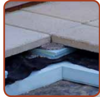
AMENITY DECK FLOORING CONCRETE PEDESTAL PAVERS
