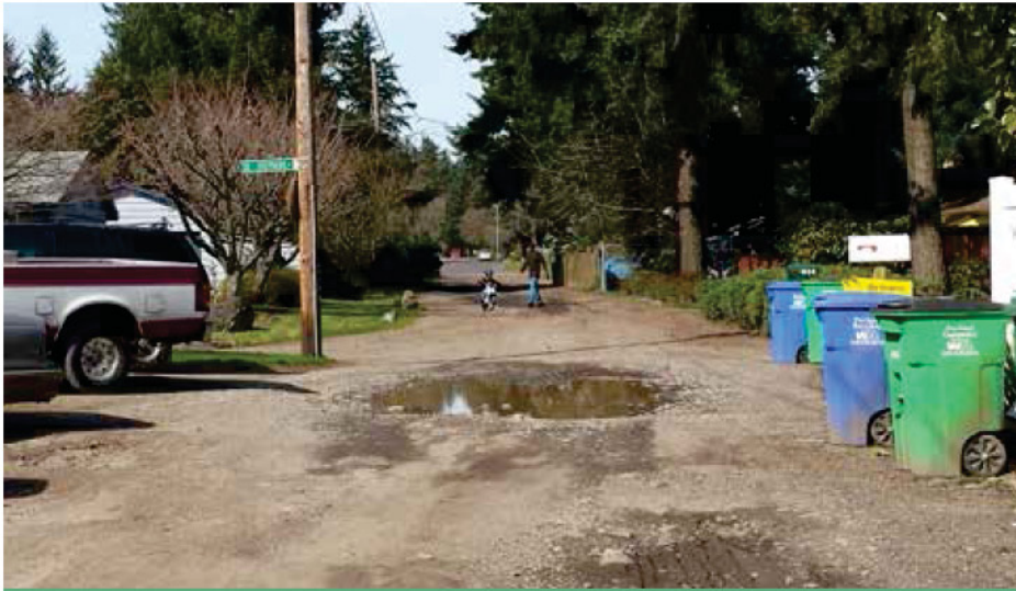
Street needing improvements
