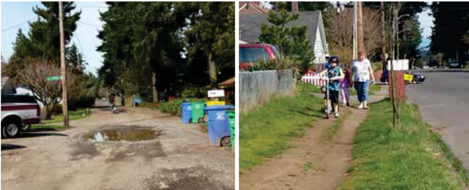
Examples of unimproved streets and sidewalks
